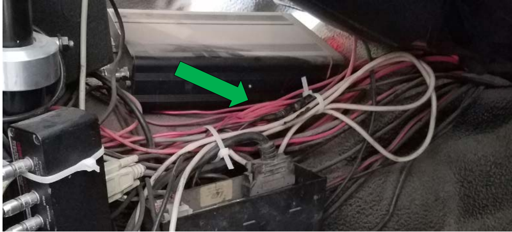
Figure 9: Example of Individual, Heavy Wires for Each Device
