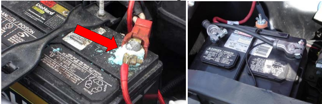
Figure 3: Examples of a Corroded Connection and a Clean Connection
